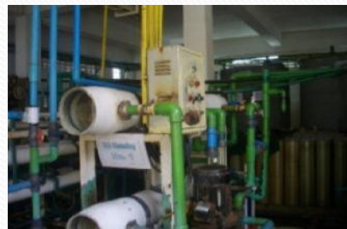
RO Cleaning Plant 2. Membrane Size 4"x40"
