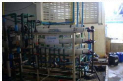
RO Cleaning Plant 1. Membrane Size 8"x40"
